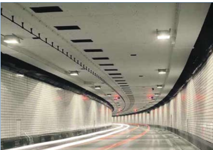
Completed tunnel project, using the Surehit to attach fire protection board and radio cable throughout.
