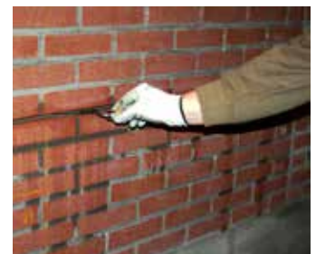
Push the bar into the grout and then inject another bead of grout
